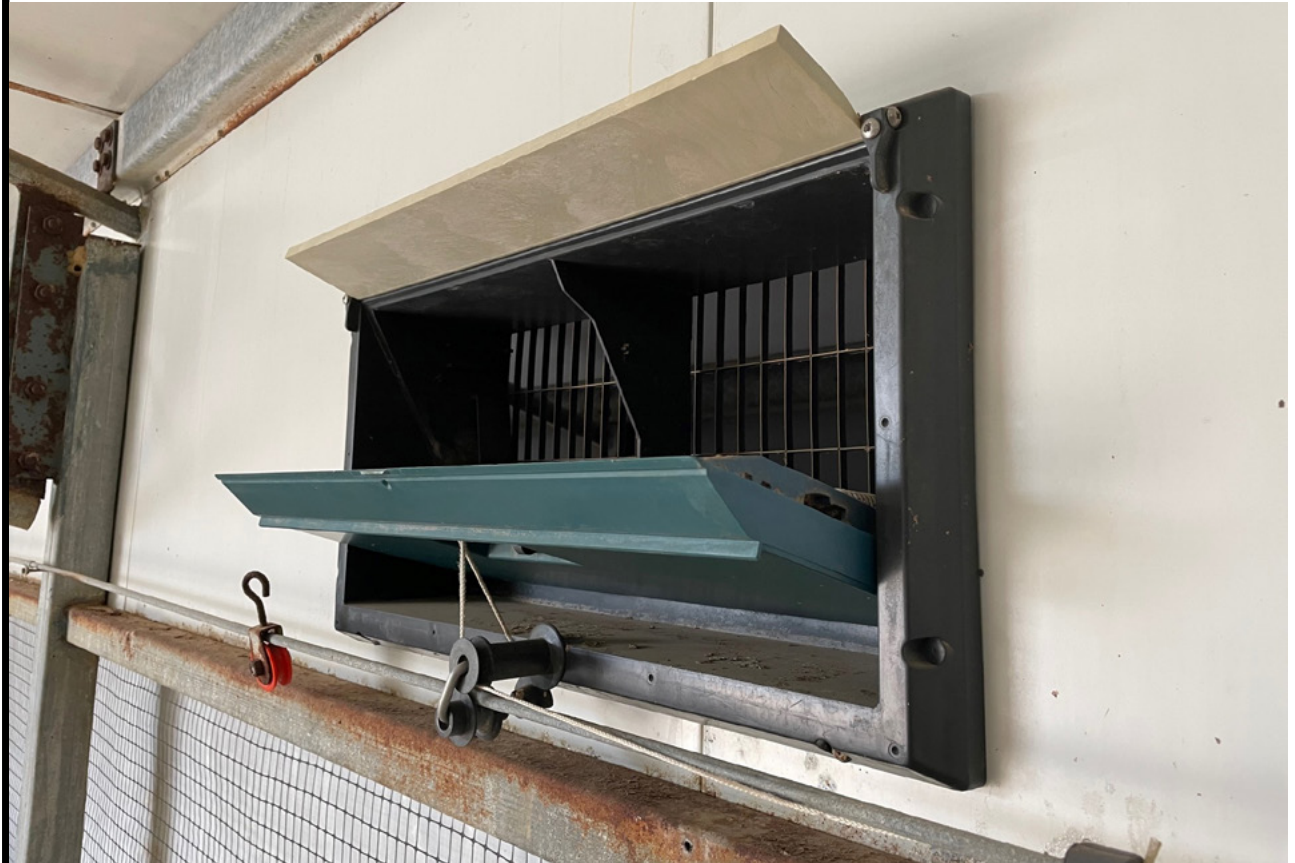
Figure 6.10 Example of a good-quality air inlet.
